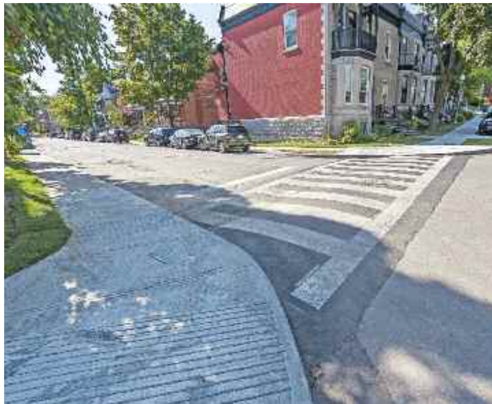
Photographed September 19, the newly reconstructed sidewalk on Metcalfe has “bump-outs” at its intersection with Springfield.
