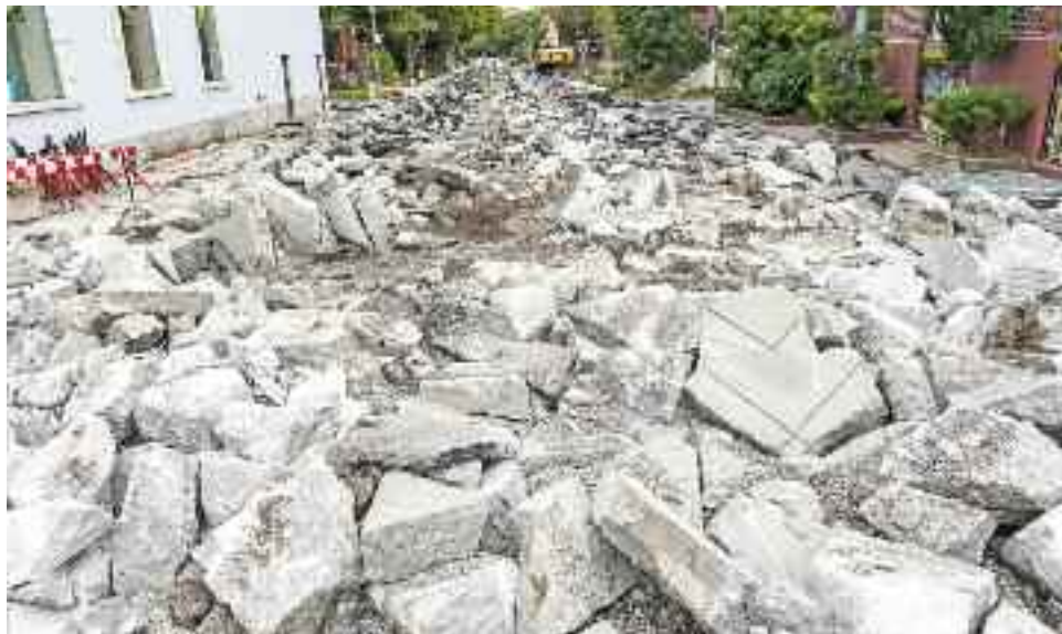
Prince Albert Ave. below Sherbrooke was a sea of broken-up concrete and asphalt September 23. The project to start the new Prince Albert public square started a week later than announced.
