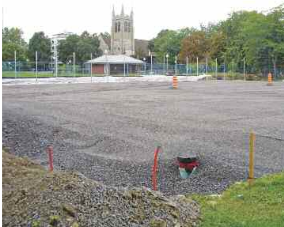
Viewed from Academy Rd. looking northwest, work to rebuild the junior tennis courts was progressing September 12. They are located just east of the underground arena.
