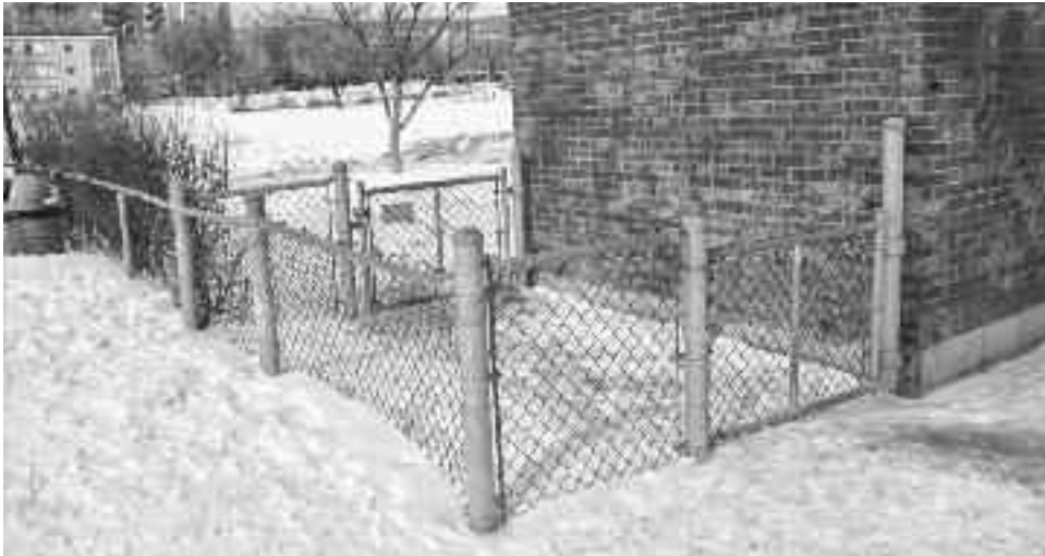
At the Westmount Athletic Grounds (WAG) dog run, snow clearance at the front entrance was satisfactory. However, the mooring of a steel post for the inner gate is breaking loose from the concrete foundation of the lavatory building that supports it.
