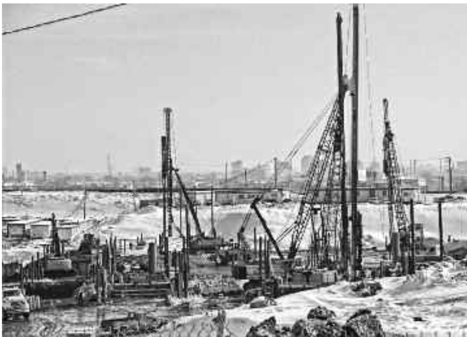
This was the scene on February 17 as piling activities continue at the incoming super hospital's Glen Yards site.
