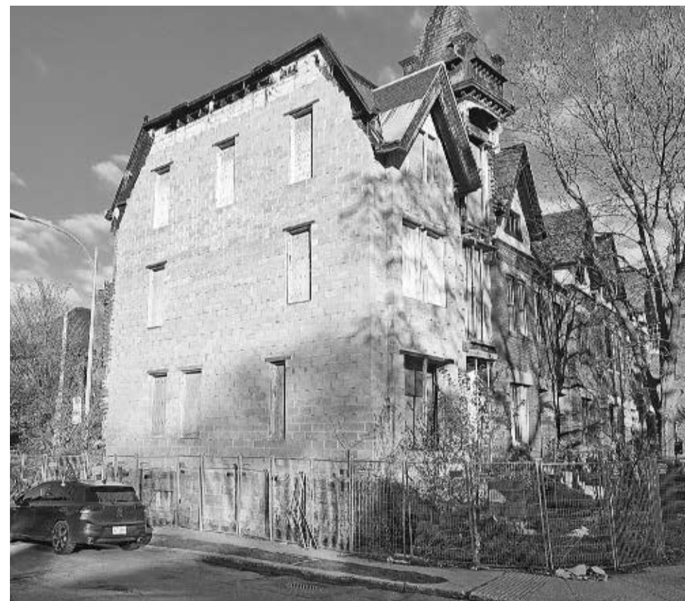
This house on Metcalfe below Sherbrooke has been under construction for at least five and a half years (see “Locked-down house?” October 27, 2020, p. RE-17), as seen May 11. PHOTO: INDEPENDENT.
