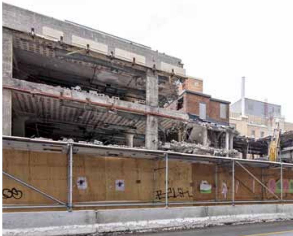
The demolition of 4014-4022 St. Catherine St. continues. It is photographed here on January 18.
