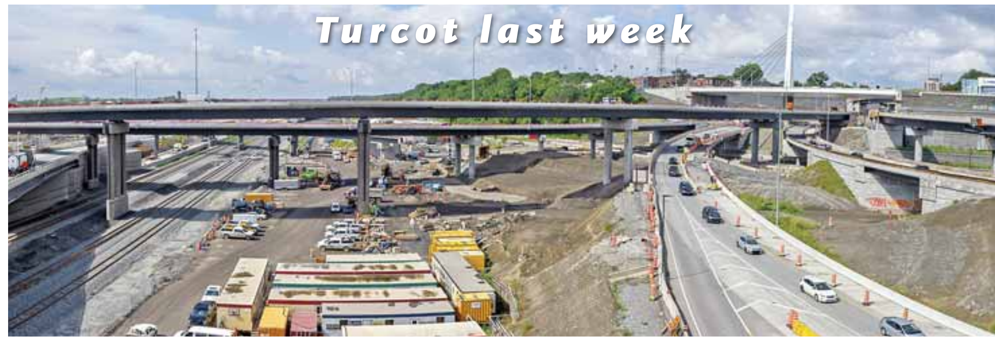
The route from Highway 15 south to the Ville Marie expressway. The new, white St. Jacques bridge over the Decarie is at top right. It was open to traffic in both directions and pedestrians when the Independent went by on August 26.
