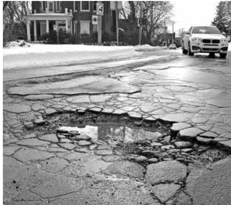
On February 17, drivers were avoiding this pothole at the corner of Claremont and Westmount Ave. or scraping the bottom of their cars going through it.
