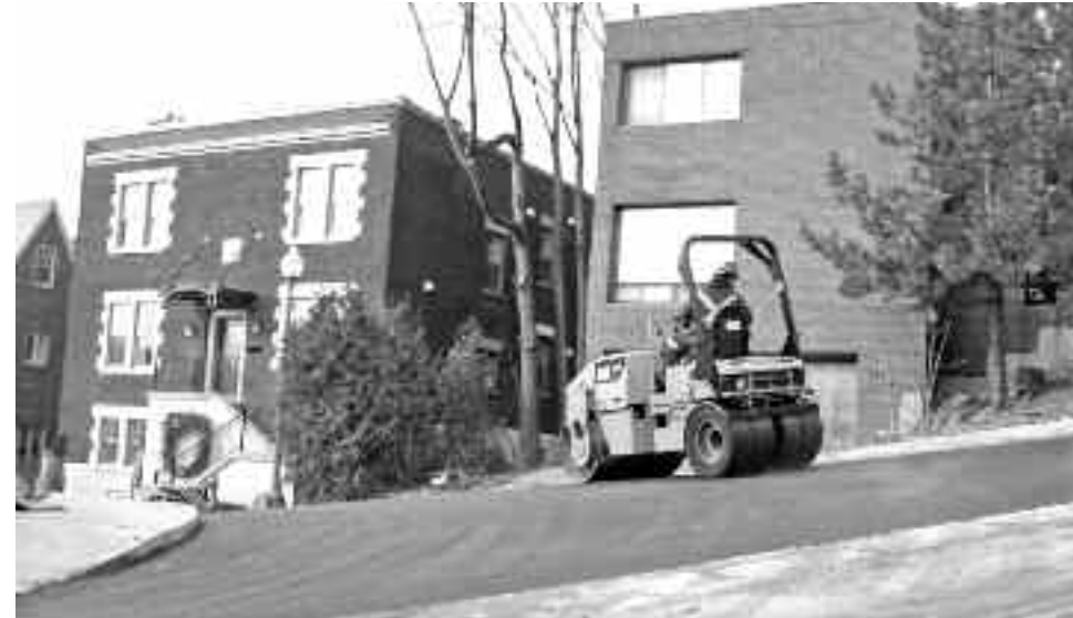
The asphalt paving of Anwoth, seen here December 8 at its northern intersection with Clarke, enabled the street to be opened to traffic after some four months.
