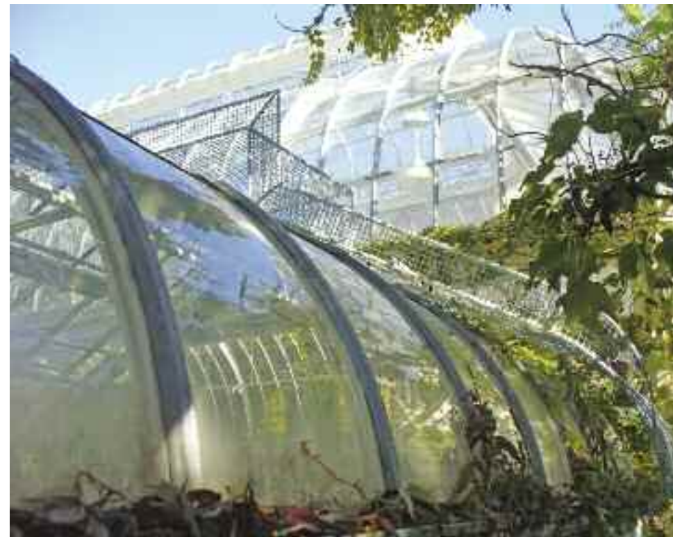
The steel structure of the conservatory is reported to be intact, seen September 29.
