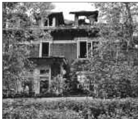
Damage from fire at 501-503 Roslyn last September.
